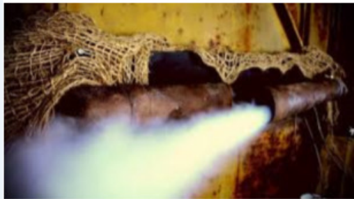
Steam line rupture (basement)
